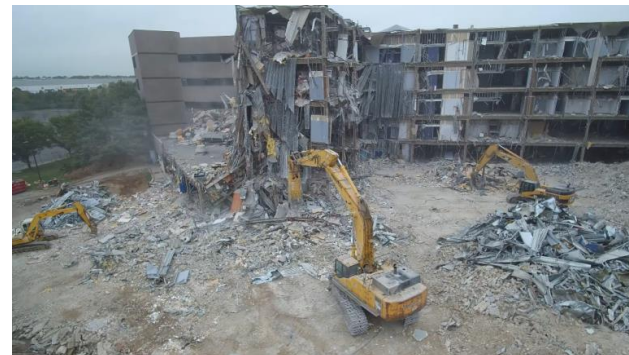
Demolishing former office building to make way for warehouse in Cranbury. Photo: Sudler Cos.
