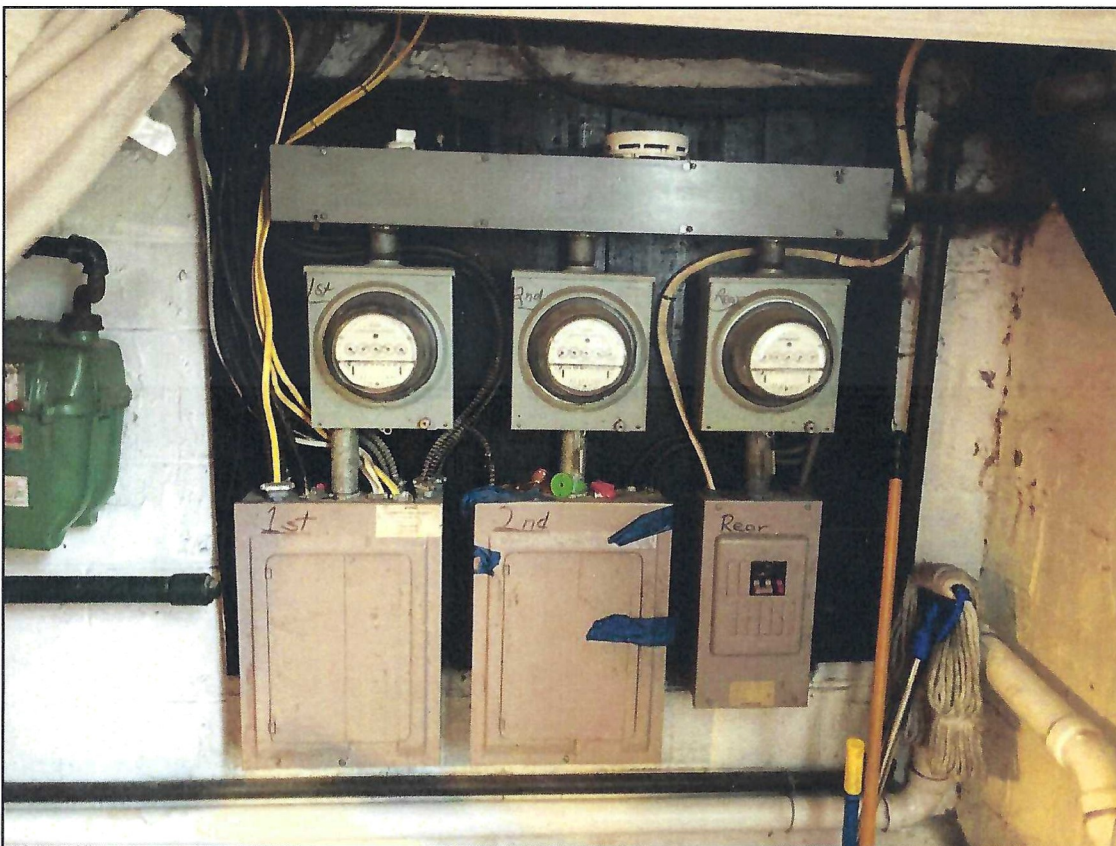
Electrical panel in basement. Not part of original construction.
