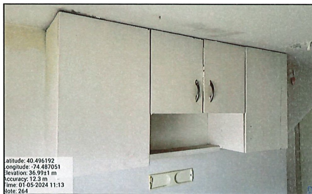
Third floor cabinets; the metal cabinets as shown above are typical for 1930s through 1950s construction.
